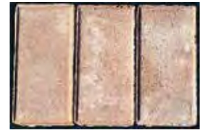
Pavers with efflorescence
